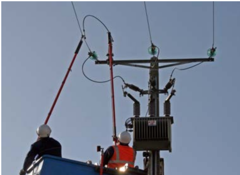
Figure 2. Utilities are improving system reliability by installing more current fault sensors on their powerlines.
